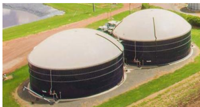
Figure 12 Example of an engineered above-ground digester
